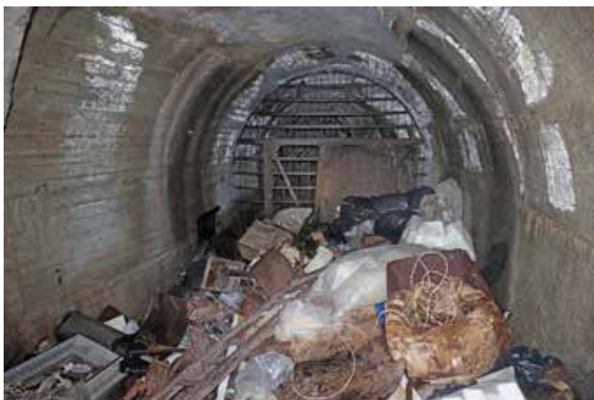
About halfway along the tunnel we were halted by a secure metal grille and beyond it a block wall
